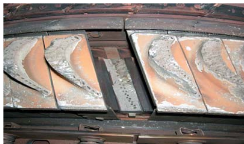
(b) Broken blade in the first row
